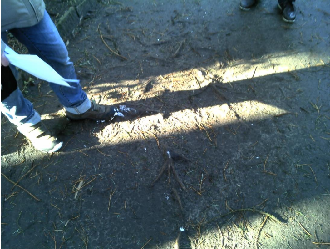
Figure 8: Roots covering a larger part of the road
