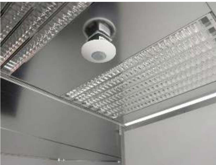
Integration of PIR and door contact sensors into the system. Monitoring of PIR signals onto a tablet PC. Gaining PIR data onto the cloud. Testing sensitivity of PIR sensors and lag time in data acquisition.
