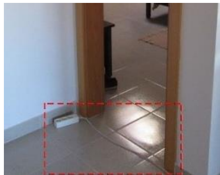
FIGURE 8 – CABLING ACROSS PASSAGE ZONES
