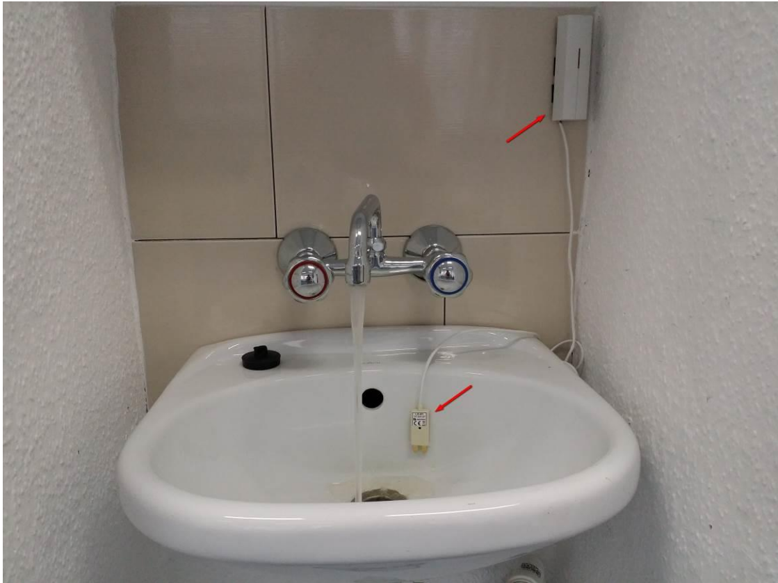
Fig. 3. PIA Integration Site – sink equipped with flood detector working with wireless transmitter.
