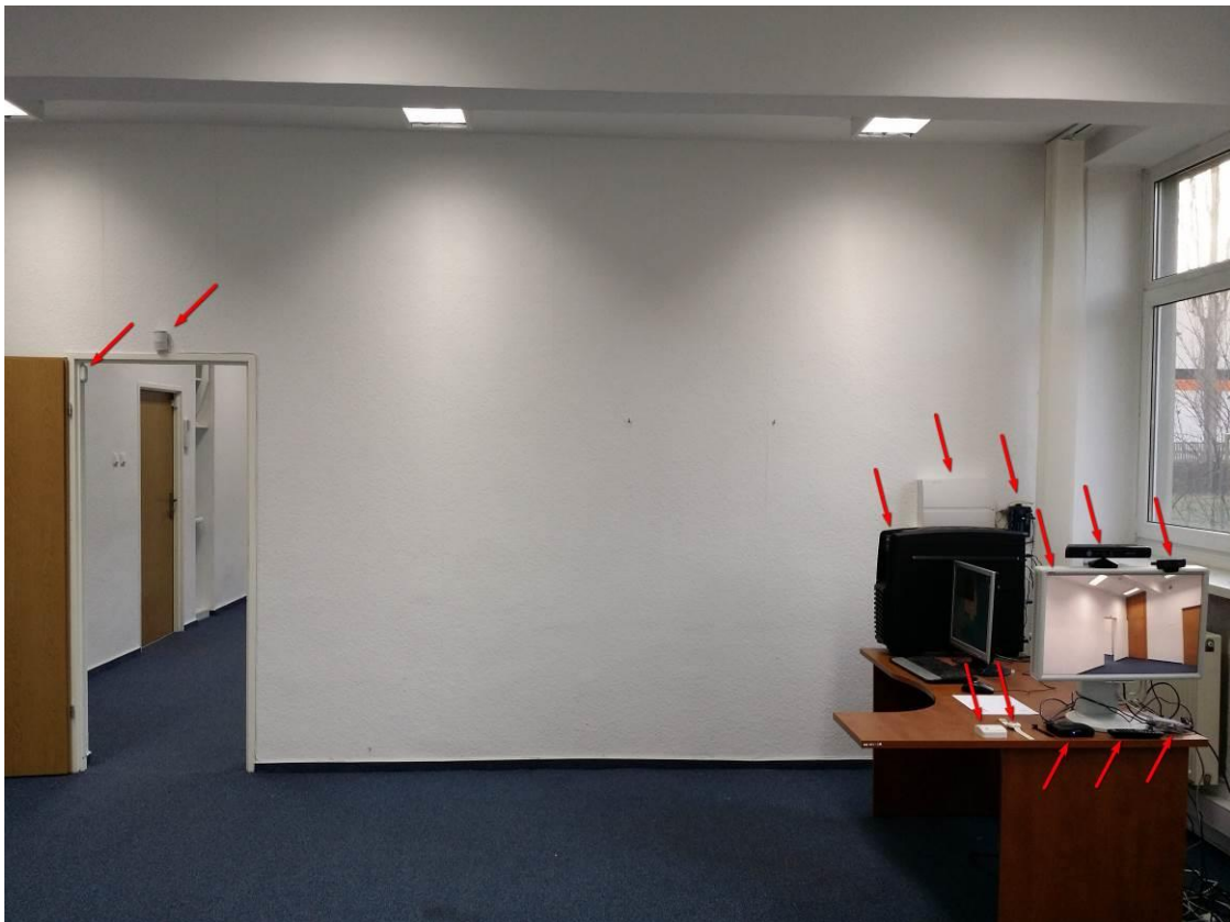
Fig 4. PIA Integration Site – Room 2 – Pose recognition server, Main Control Unit, Moxa Nport server, wireless & wire movement detectors, MS Kinect, Raspberry Pie unit, Logitech HD camera, wrist emergency button, wall programmable button.
