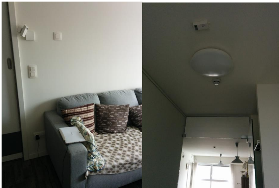
Figure 5: Examples of sensors installed in the flat.
