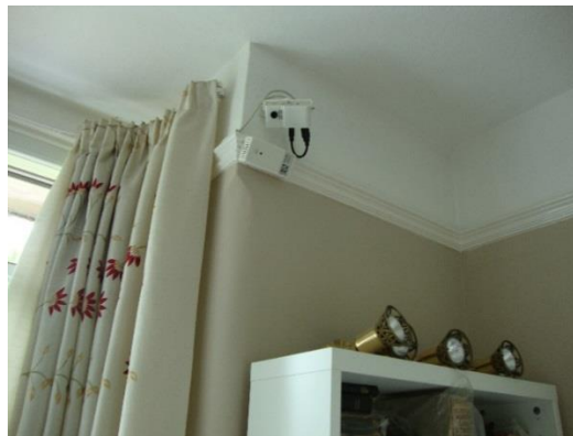
Figure 8: Picture from installation in Surrey
