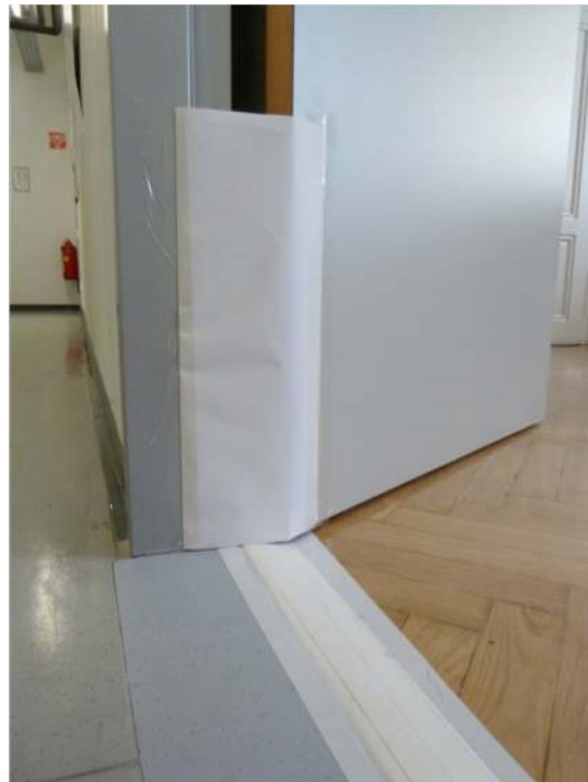
Figure 17 Clearance between door frame and door leaf
