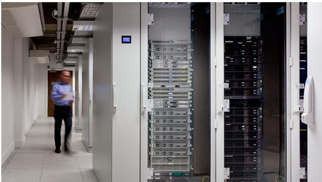
Figure 24 Data Centre Interior
